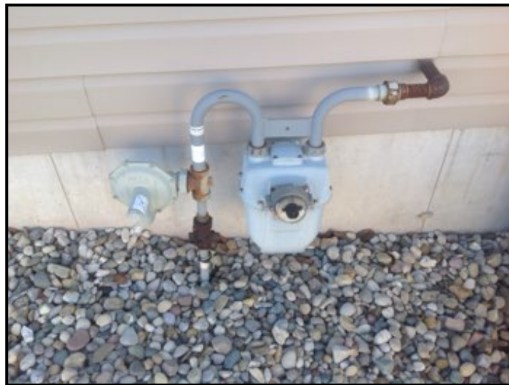
Surface rust present.
