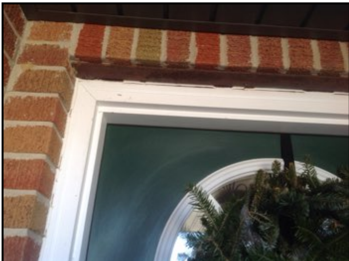
Front door needs caulked.
