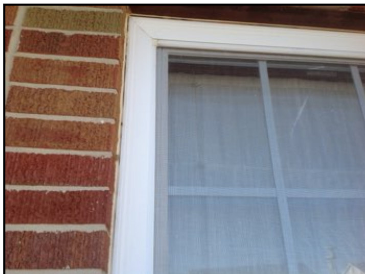
Windows require caulk.
