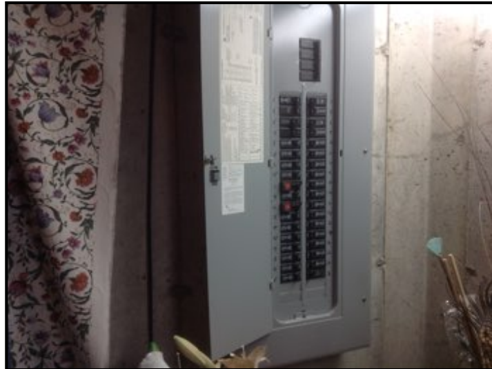
GE panel present. Circuits are clearly marked.
