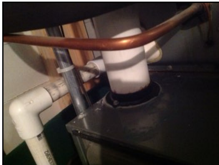
Some surface rust noted.
