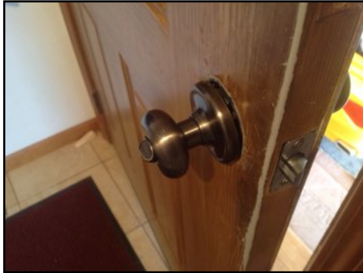
Lock set on door to garage needs repaired.
