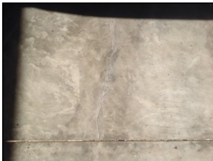
Some surface cracks noted.
