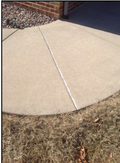
Expansion joint in front sidewalk should be caulked to prevent water intrusion.
