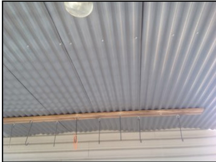
Unable to inspect underside of deck due to deck ceiling installed.
