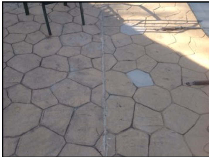
Patio shows evidence of mud jacking. Keep maintained and sealed to avoid water intrusion.
